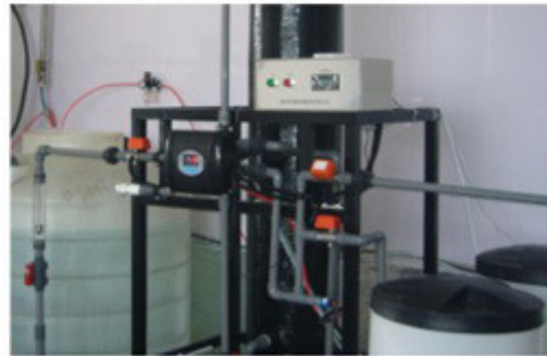
○高纯水处理设备 High Purity Water Treatment Equipment
