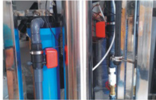
○反渗透预处理 The pretreatment of reverse osmosis
